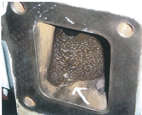
Corrosion of exhaust gas pass of Cylinder Head
